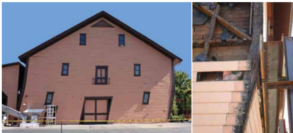
Figure 2. Post-earthquake deflection and localized damage at second-floor level.
