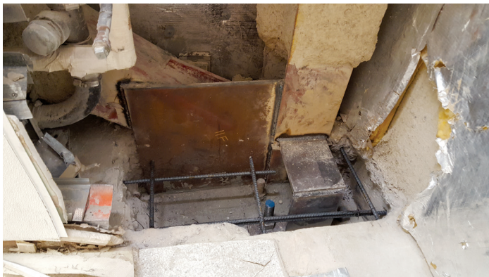
Figure 1. Base of existing braced frame column retrofitted with new gusset plates and anchor bolts.
