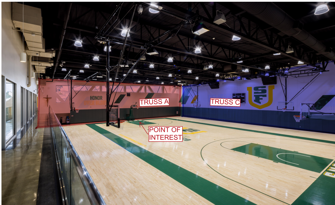
Figure 22: Interior of Finished Gym Looking North, Showing "Point of Interest" for 3D Vibration Analysis
