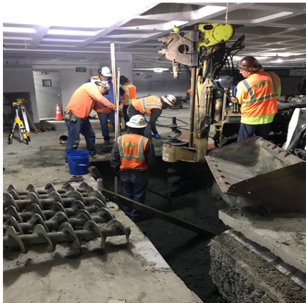
Figure 18: Low-Overhead Drill Rig to Install Micropile Foundations at the Bottom Level of the Existing Parking Garage
