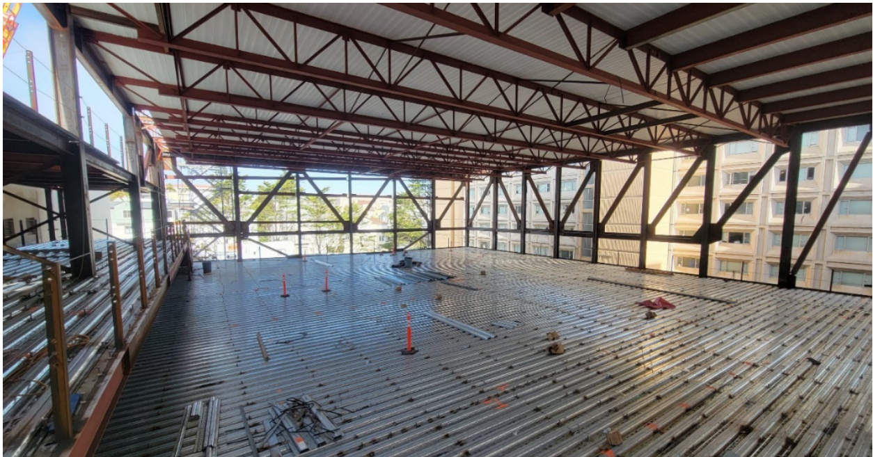
Figure 5: Custom Open Web Roof Joists Over the Main Gym Floor; Truss A at the Far Wall, Truss C to the Right
